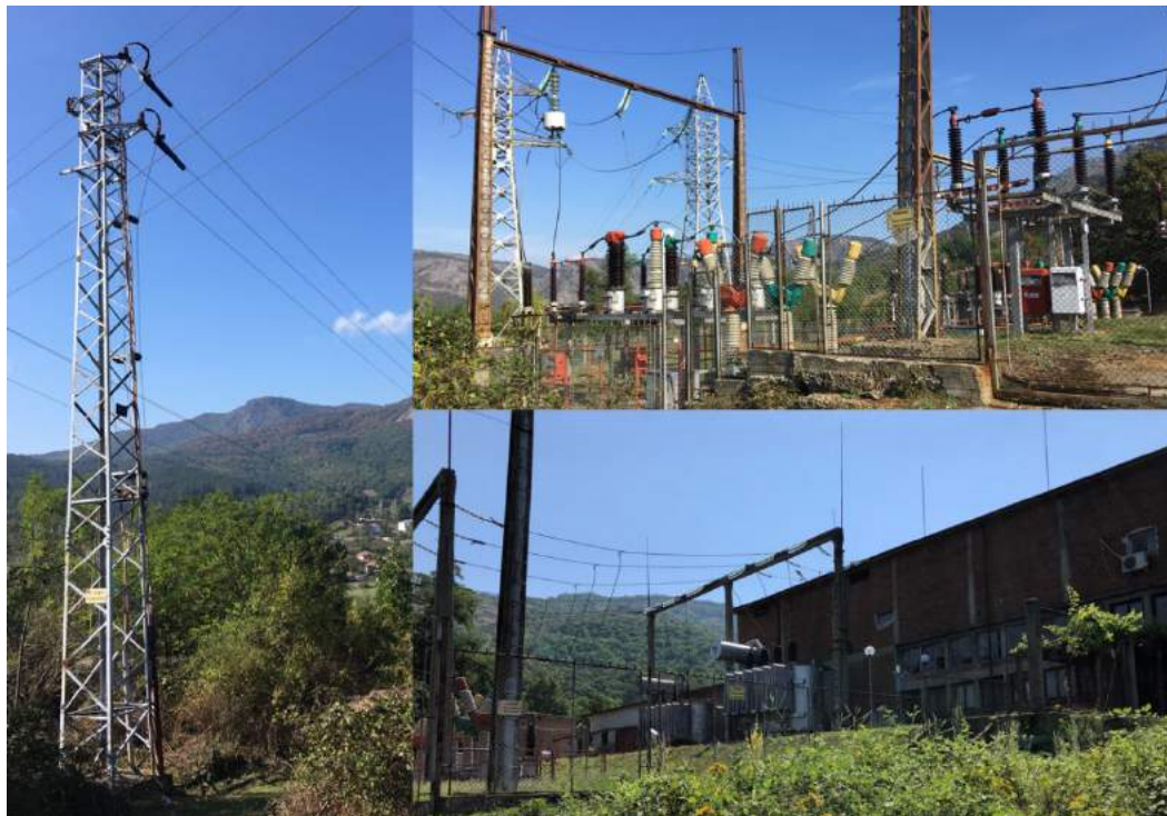
Figure 18-4 : Pylon to support a 110 kV power line and the Madzharovo substation.
