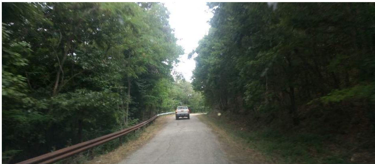
Figure 18-2 : Existing sealed access road between II-59 and the Rozino Project site (Source: Velocity, 2020)
